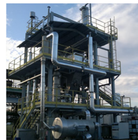
2008- Internal recirculation Bubbling Fluidized Bed reactor-500 kWth (ICBFB)
