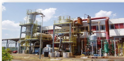
Integrated pretreatment and fractionation station (300 kg/h wet biomass) Mossi & Ghisolfi 2012 – now ENI-Versalis
